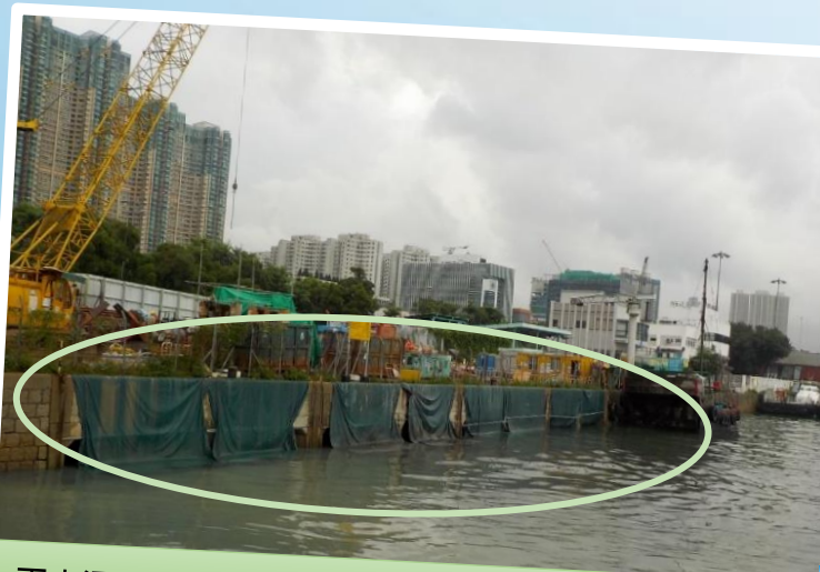
雨水渠出水口加裝帆布 Canvas sheets are installed at the box culvert outlets
