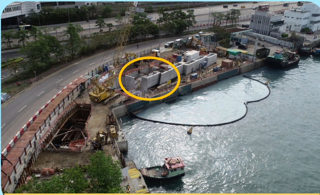
用預製組件興建旱季截流器的維修走廊 Constructing the Maintenance Corridor of DWFI by prefabricated concrete modules
